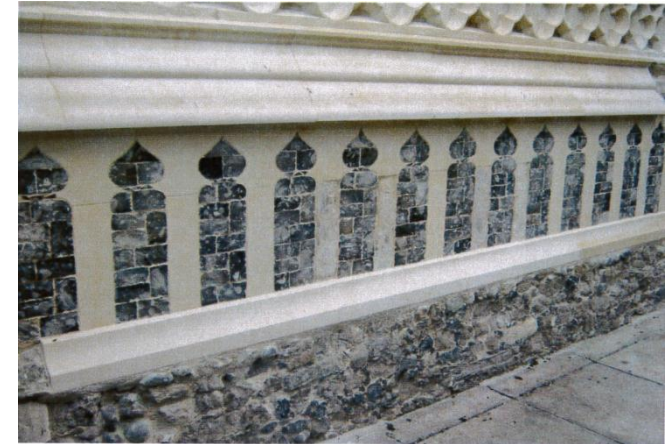
Award winning flint work and masonry repairs carried out on St. Lawrence Church, Ipswich
