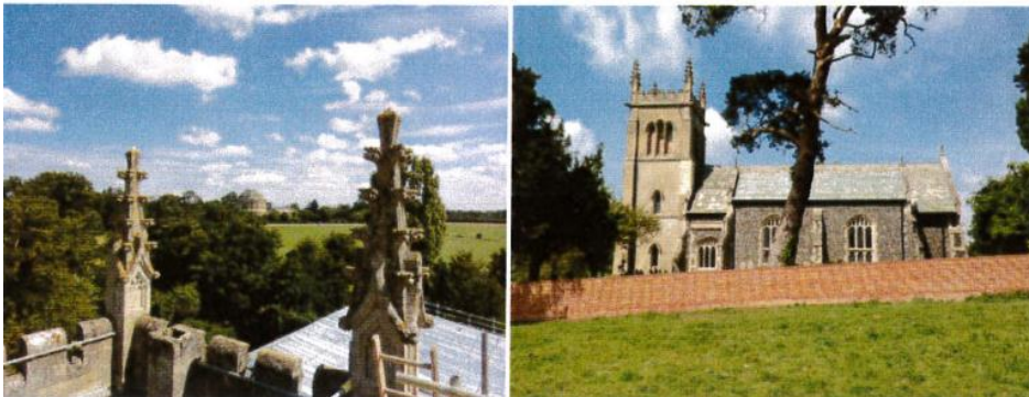
Award winning major restoration of Grade II listed St. Mary's Church, Ickworth, Suffolk
